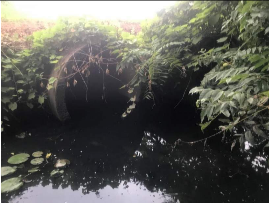
Photograph No. 13 STA 11+50 Upstream photo of 48" RCP with twin pipe next to it
