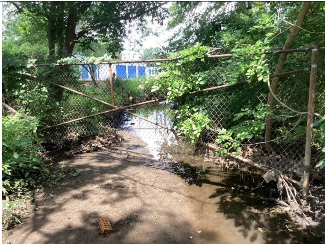
Photograph No. 4 Fence Obstruction along Main Channel Stream
