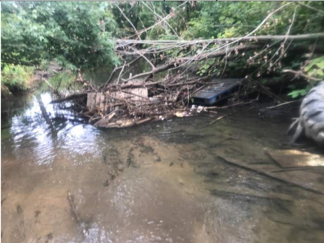
Photograph No. 60 41°2'24" N 81°26'6" W Downstream photo of buildup in creek
