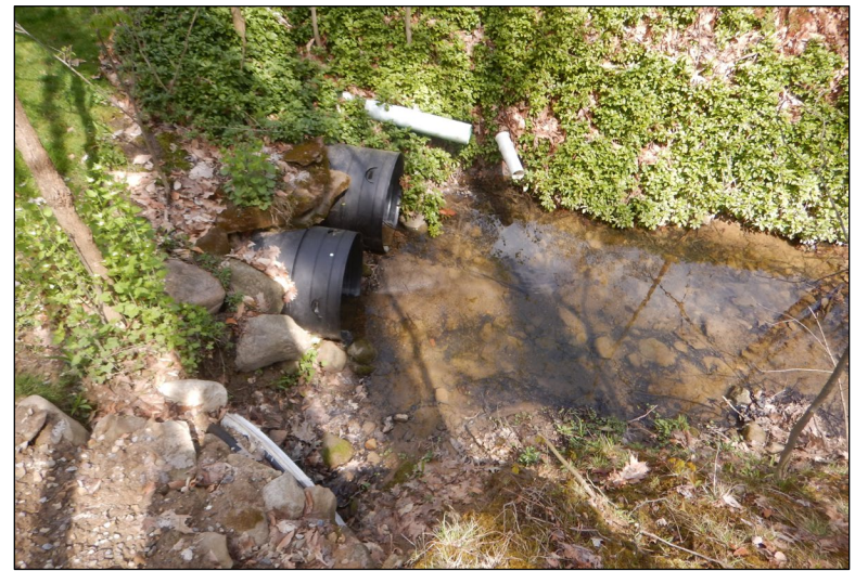
Photo 54: View of the culverts on the west side of Stream 3, facing north.
