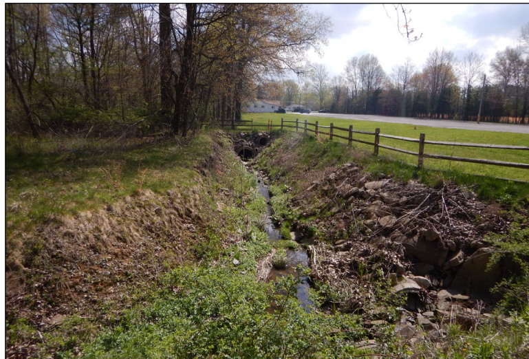
Photo 39: View of the culverts west of the VFW, north of the parking lot that carry Stream 1 under the parking lot to the south. Photo facing east.
