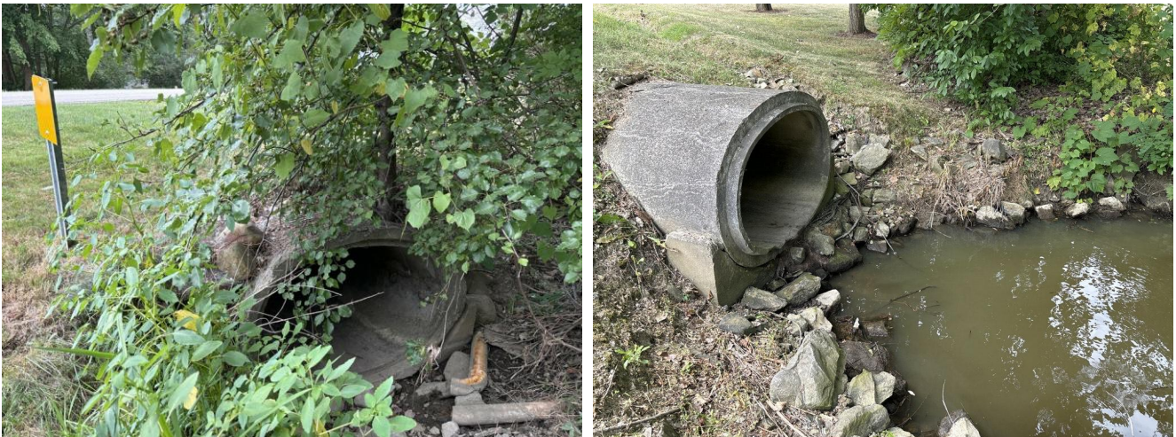
Figure 1. 53" x 34" elliptical concrete culvert under Chaffee Road, looking at upstream end of culvert (left) and downstream end of culvert (right)
