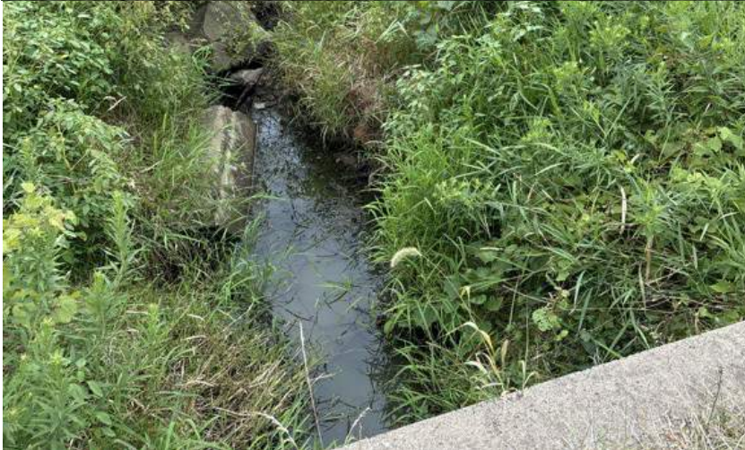
7720 Carter Rd Limited buffer next to driveway w/ no trees Looking D/S
