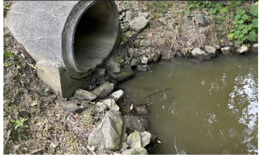
Chaffee Rd Culvert = 53" x 34" (elliptical) Scour hole present D/S end
