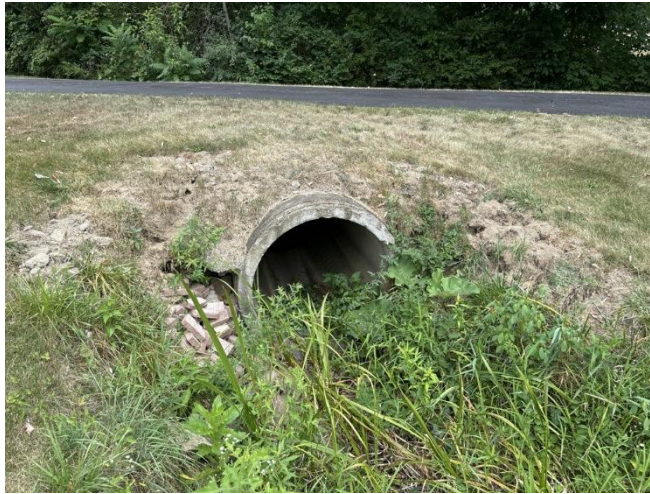
Figure 2. 42" concrete culvert under the driveway of 7565 Chaffee Road, looking at upstream end of culvert
