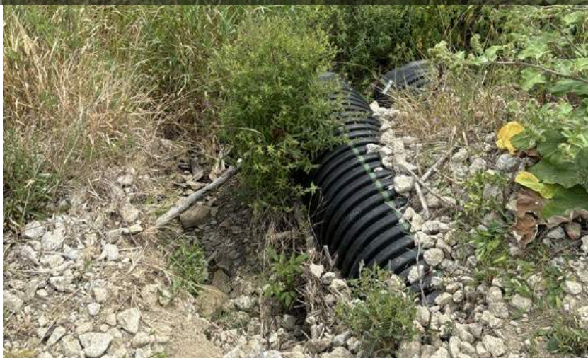
7495 Chaffee Rd culvert (CEI parcel) = Two 24" Inlet has erosion and lacks armoring U/S end
