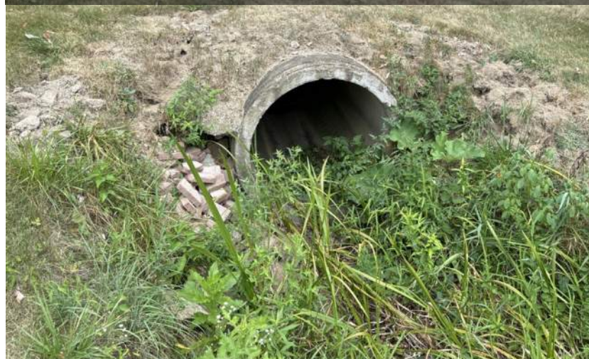
7565 Chaffee Rd driveway culvert = 42" Erosion evident around sides U/S end
